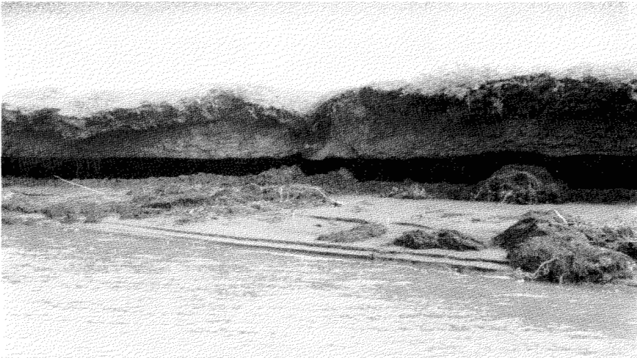
Fig. 3. Exposed undercut along right bank of the Colville River.
