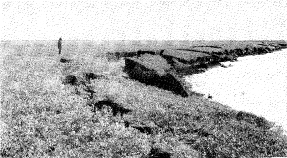
Fig. 2. Collapse of right bank through action of high waves generated by westerly winds.
