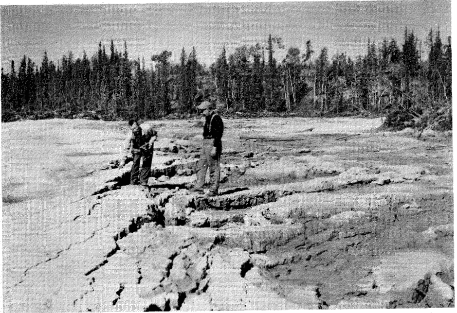
Fig. 1. Thawing of frozen soil following clearing for road construction; the soil was a fine silt with such a high moisture content that it slumped and flowed as it thawed, once the vegetation cover was removed.
