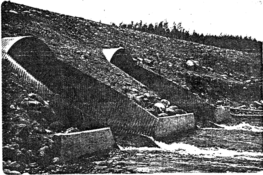
Plate 5: Poplar River culverts: rapid water flow and elevated outlets obstruct fish passage.
