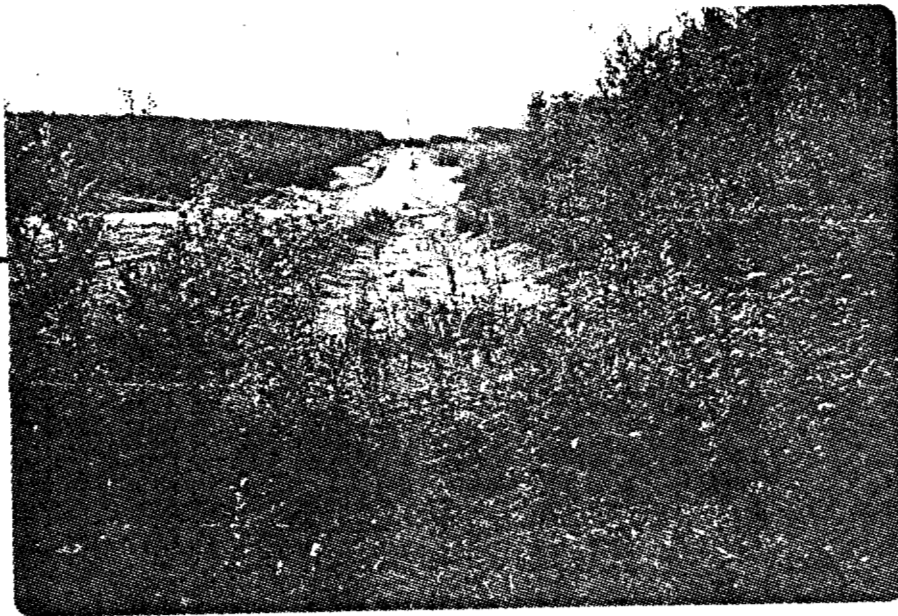
Plate 3: Ditch block to direct water into cross drainage culvert, and offtake ditch. This ditch block has apparently been placed incorrectly, resulting in clogging of the culvert (plate 4).
