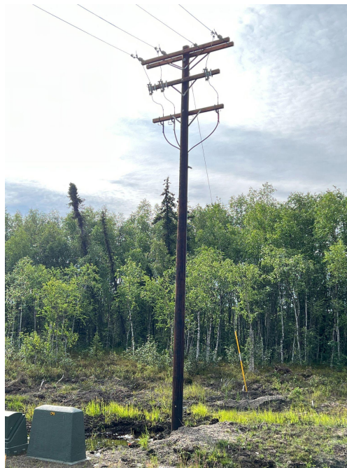
Power pole 641 in Galena, AK. Photo Courtesy of Kartorium
