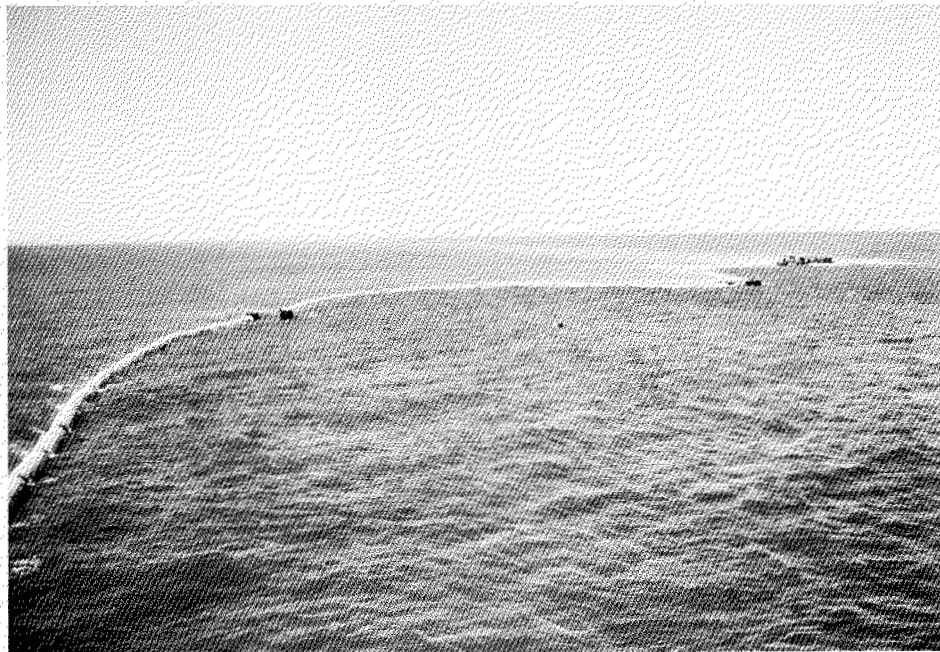
Plate IV Turbidity plume from construction of Isserk F-27. This view is from the suction dredge Beaver Mackenzie, July 26, 1977.
